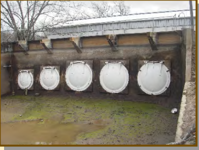
● River Plant Discharge Gates
