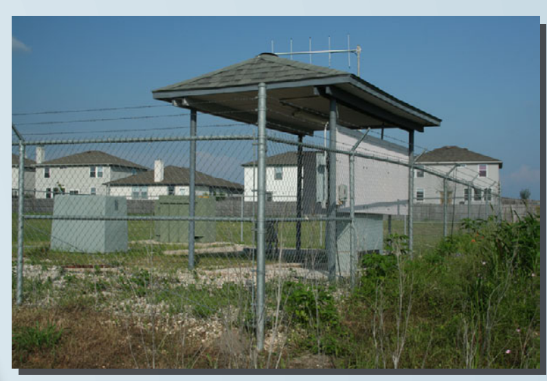
Photo 10. Automated sewage lift station in Wild Horse Ranch subdivision in Manor.
