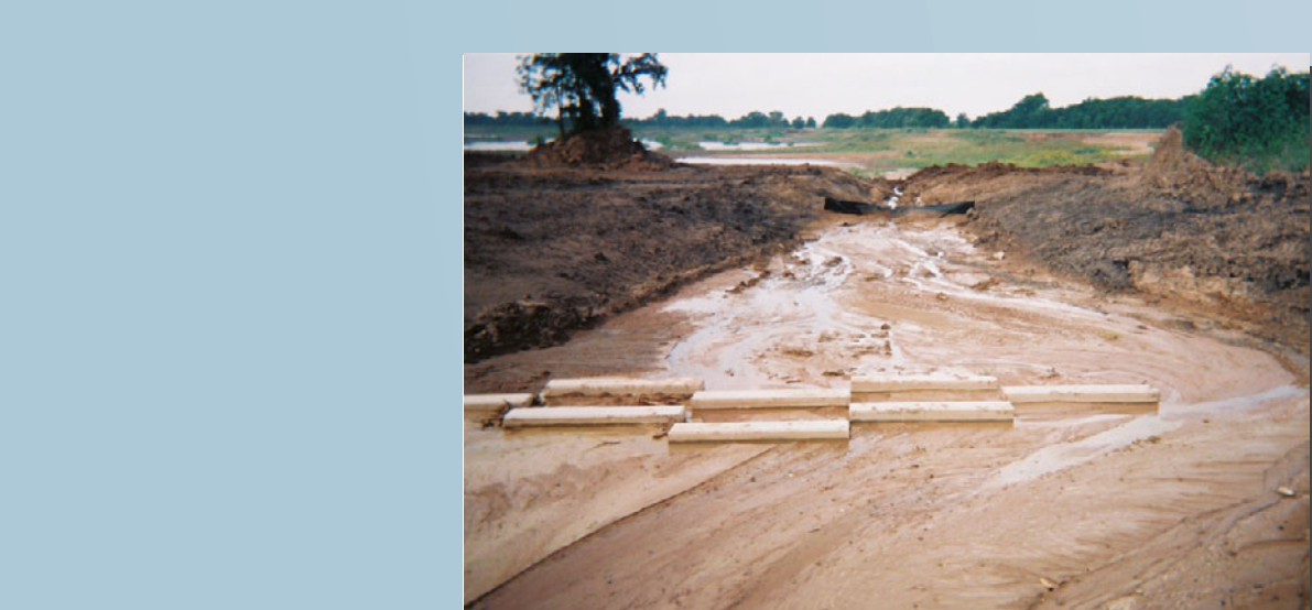
Photo 13. Sediment-laden runoff from SH130 road construction near Hornsby Bend.
