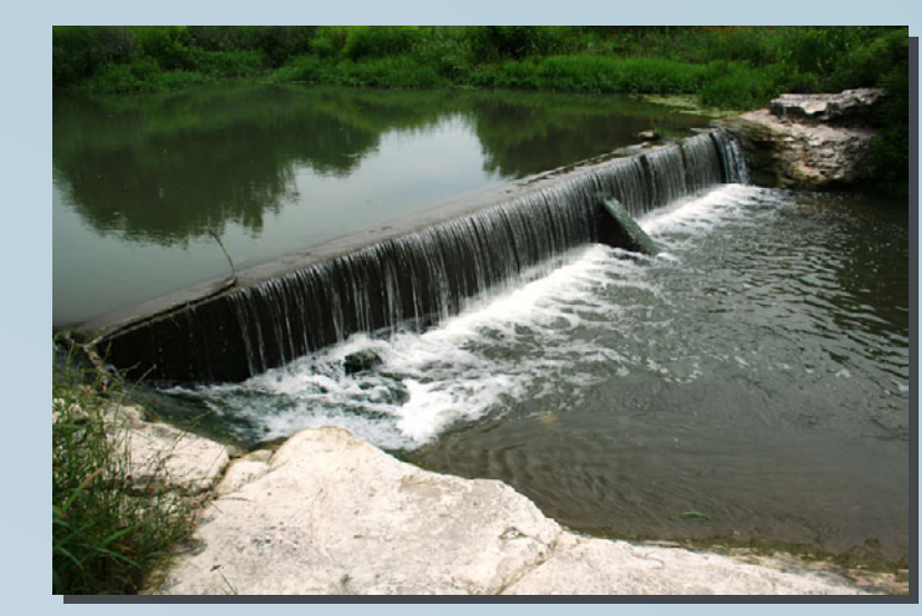
Photo 3. Concrete weir in Gilleland Creek downstream from Swenson Park Boulevard in Pflugerville.
