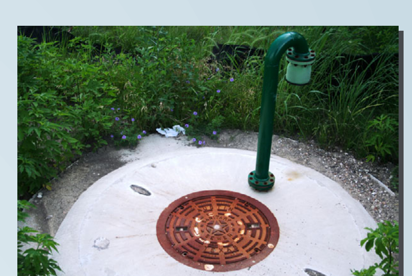
Photo 9. Sanitary sewer near Gilleland Creek in Ben E. Fisher Park in Manor.
