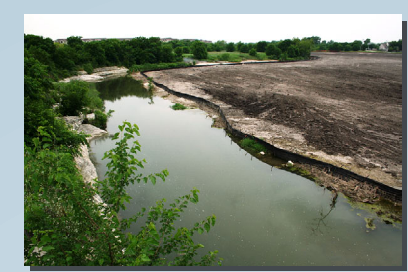
Photo 2. Riparian area under construction from bridge on Swenson Park Boulevard in Pflugerville.
