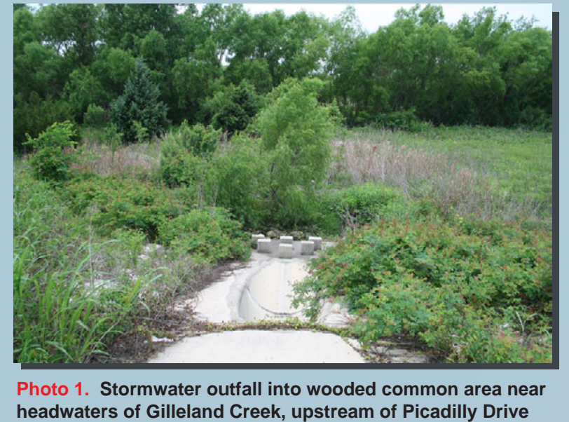
Photo 1. Stormwater outfall into wooded common area near headwaters of Gilleland Creek, upstream of Picadilly Drive in Pflugerville.
