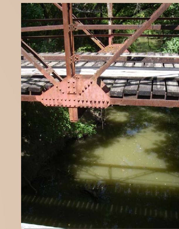
Photo 7. A trellis bridge crosses over a deep stream channel of Wilbarger Creek at Upper Elgin Road. This is a downstream view.
