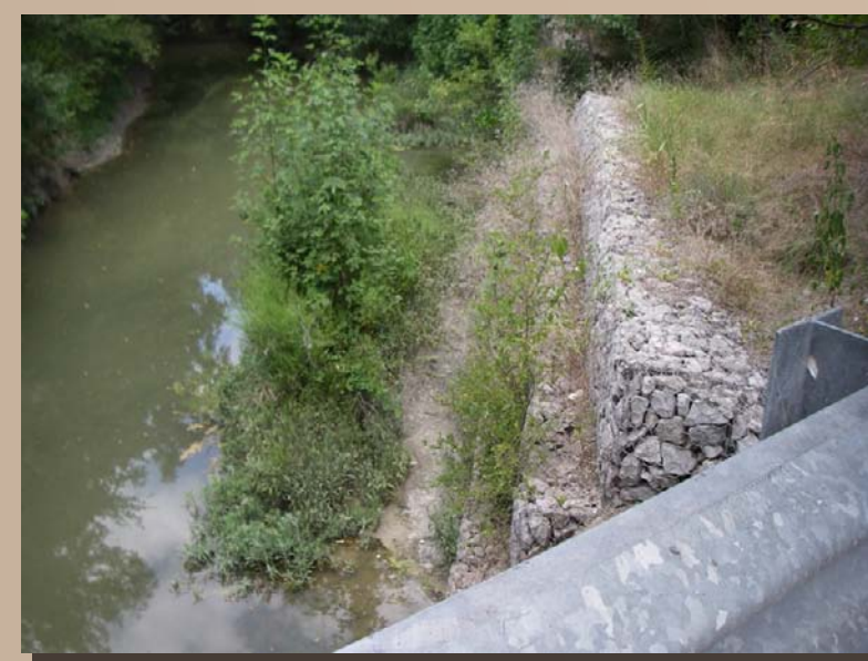
Photo 4. As this upstream view shows, gabion stream bank protection is built along Wilbarger Creek at Jones Road.
