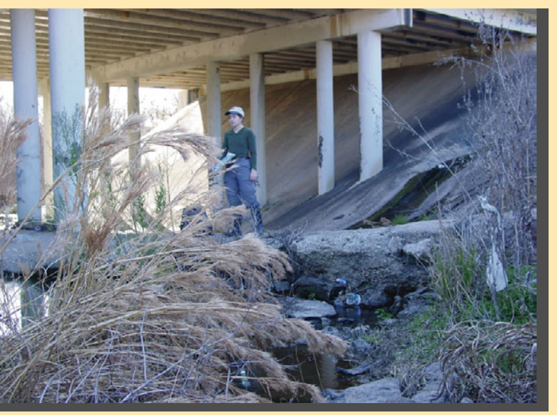
Photo 16. FM 1431 Bridge, upstream side, exposed wastewater line in concrete encasement, creek has scoured below the wastewater line.
