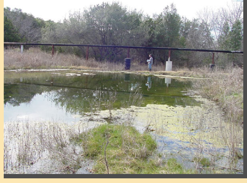
Photo 31. Extension of Bridget Lane, looking downstream at elevated wastewater line above creek, crossing is creating a pond.
