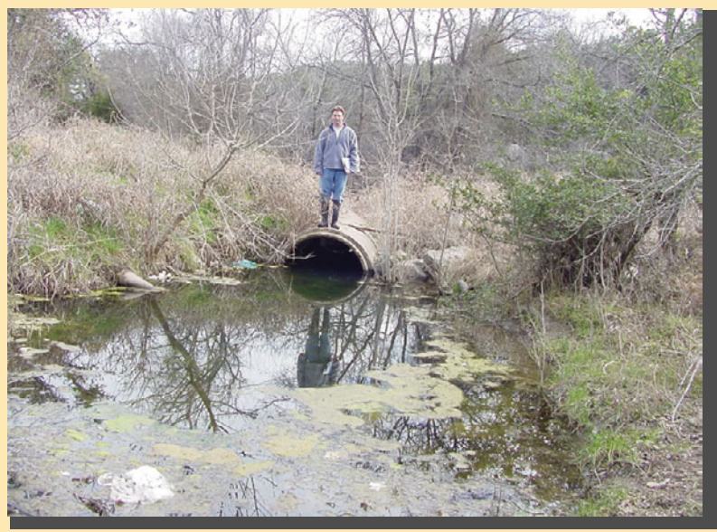
Photo 29. Looking downstream at culvert across creek, notice trash and algae, flow is impeded.
